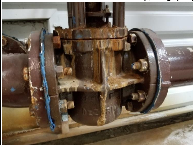
Valve plug, suction sludge pump BW Tank No. 2 (Score: 4-Poor)
